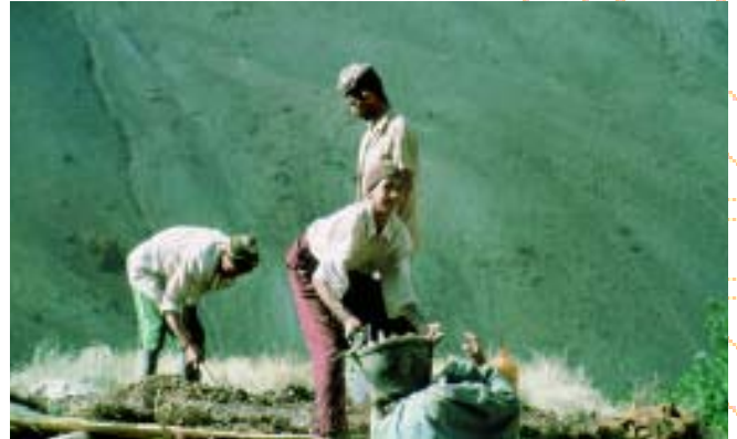
In the High Atlas Mountains (Morocco), local construction materials are used: earth, stone and wood. Terraces are made of layers of earth, firmly compacted with a special wooden implement (marcaze). To maintain their impermeability, the women go out on the terrace when the earth is moistened by rain and dance, often accompanying themselves with song. © X.Casanovas I Boixereu
